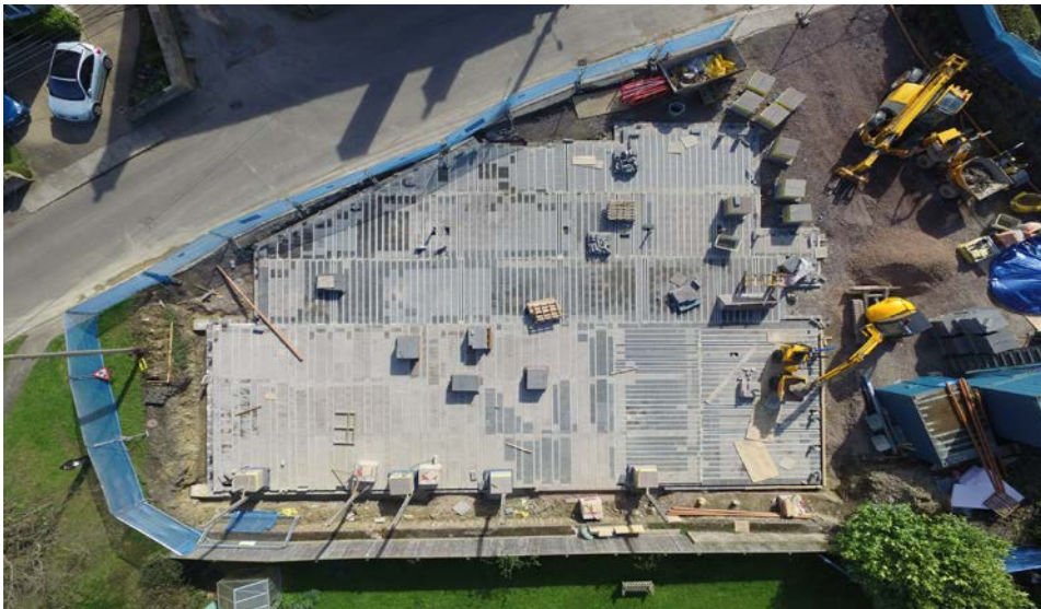
Photo 1. Aerial Photo showing ground floor installation
